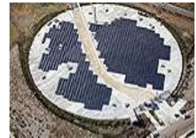
Photovoltaic system at Alvarado Water Treatment Plant
